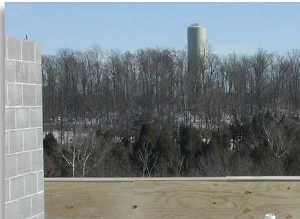
The distant elevated water tank above this roofline has been sized to meet the Insurance Services Office Needed Fire Flow formula for this project.
